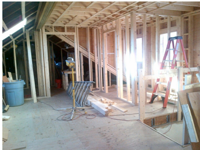
64 Hooker Ave – dormer under construction from street (top), neighbor's rear yard (middle), inside house (bottom)
